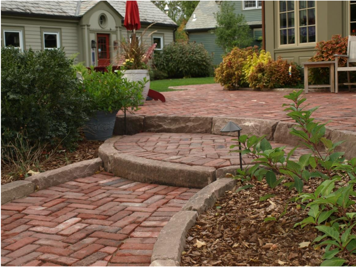
Radiused Medina curbing create edging for the reclaimed street brick paver walkway, step, and patio.
